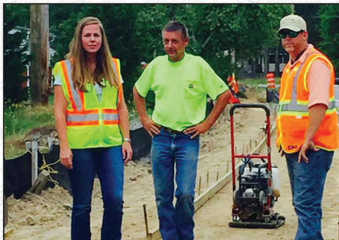
Kristen Orton, Jimbo Brown and Jason Bridges at West Sandtown Road sidewalk project.
